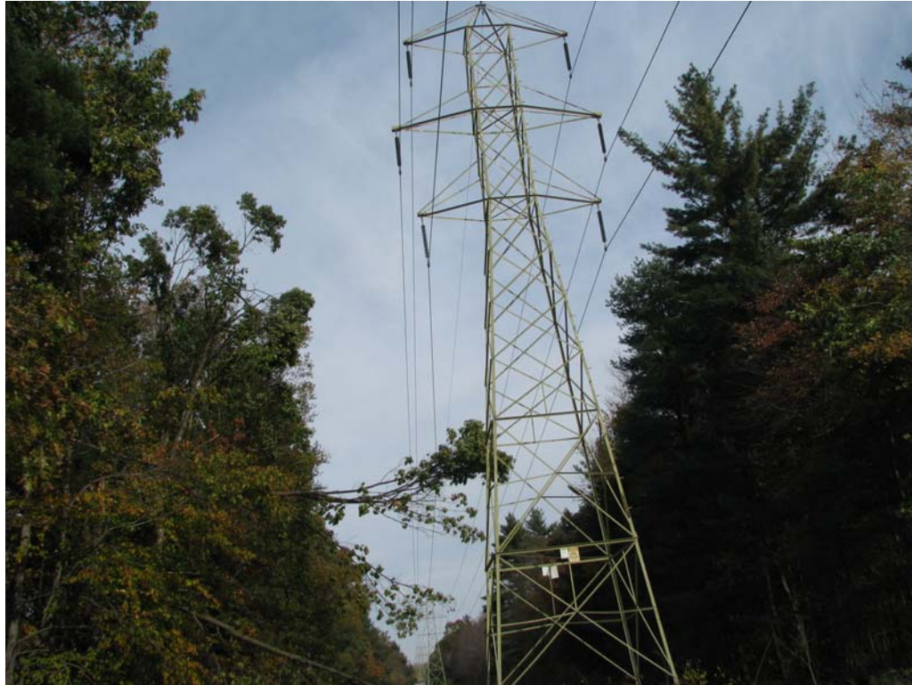
Figure 14: Tall Tree Fallen on an 115kV line in Massachusetts
