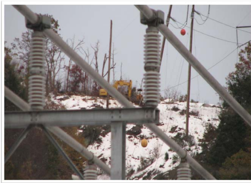
Figure 15: Structure Failure on a 345kV Line in Connecticut
